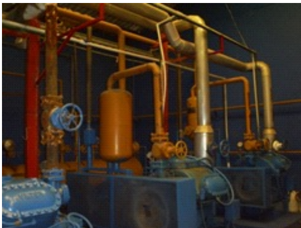
illustration 1: Before: piston compressors area of refrigeration system
